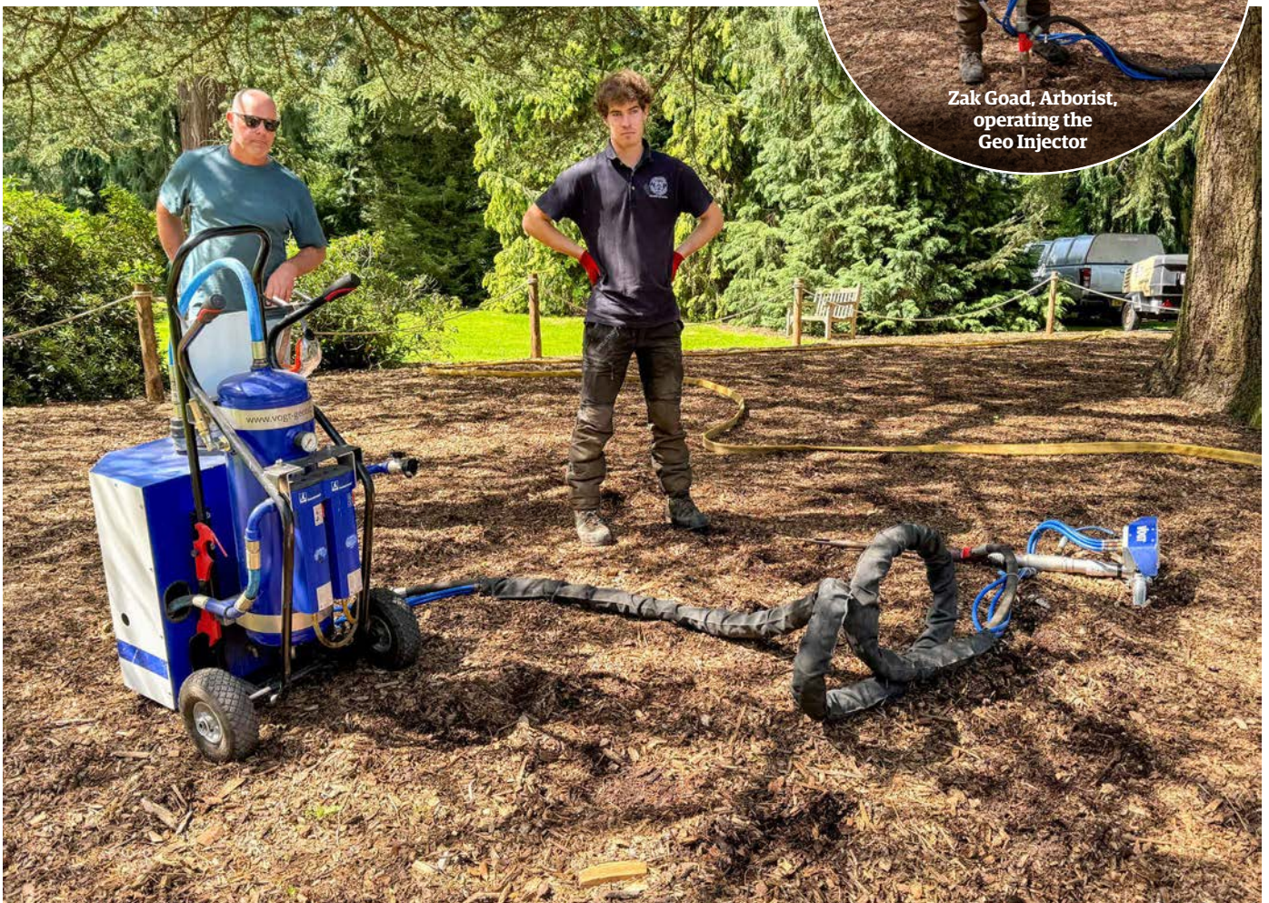
Geo Injector configured for decompaction work with Mike Harvey, Arboricultural Supervisor and Arborist Zak Goad
